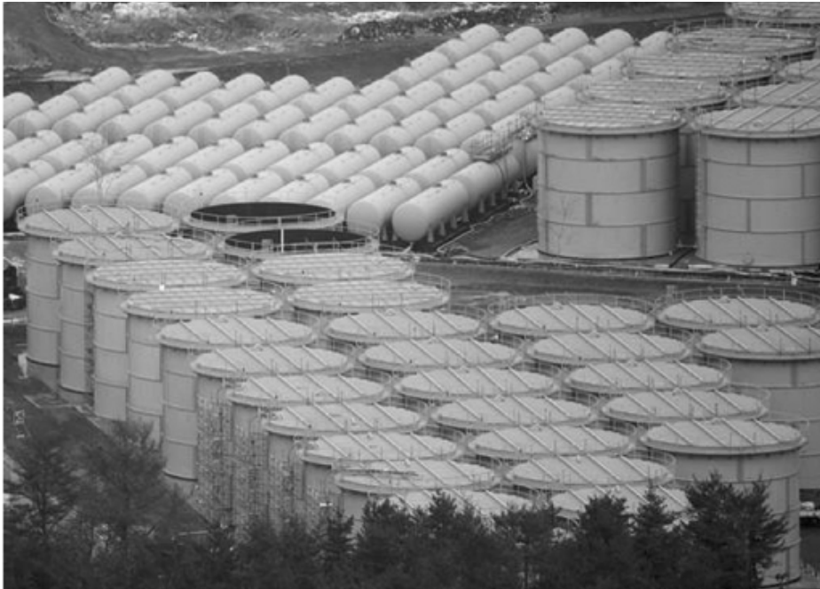
(a) An image of a tank array in the FDNP [92].
